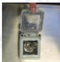
The key switch is placed in a watertight box
